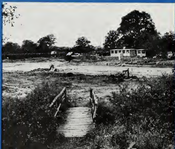
Beginning excavation where the tennis court and bowling green once were located
